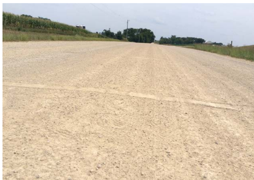
Figure 21. Control Section after scrape test
